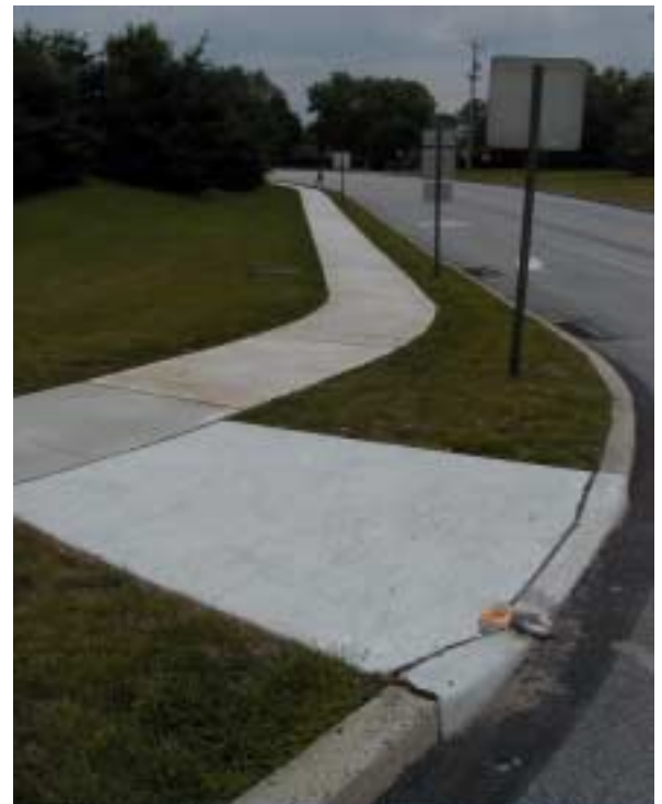
ADA curb ramp leads into prohibited crossing!
